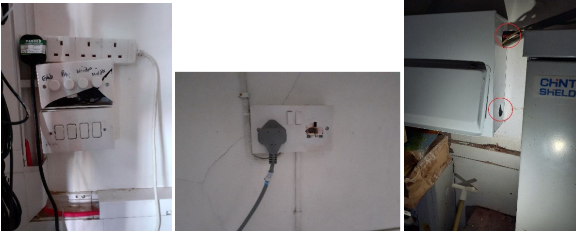
Photographs above show a broken light switch, burnt socket and gland covers missing on a distribution board.
