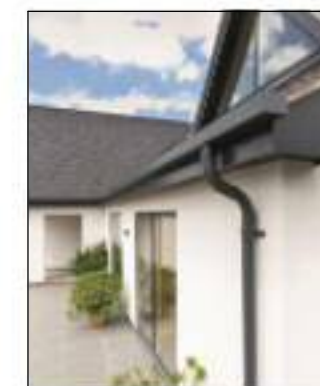
Roofing to be replaced with Riven Edgemere Concrete Interlocking Tile, in Anthracite MA35138, alongside the replacement of fascias, gutters and soffits in coordinating RAL7016 'Anthracite Grey' finish.
