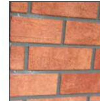
New Soltherm External Wall Insulation (Deco W-Brick ID) with brick cut render infills
