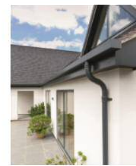
Roofing to be replaced with Riven Edgemere Concrete Interlocking Tile, in Anthracite MA35138, alongside the replacement of fascias, gutters and soffits in coordinating RAL7016 'Anthracite Grey' finish.
