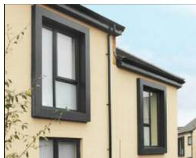
Aluminium window pods, matt finished in RAL7016 'Anthracite Grey', Windypods or similar, to be installed as per manufacturer's specifications. See detail SD511.
