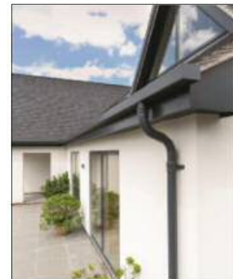
Roofing to be replaced with Riven Edgemere Concrete Interlocking Tile, in Anthracite M35138, alongside the replacement of fascias, gutters and soffits in coordinating RAL7016 'Anthracite Grey' finish.
