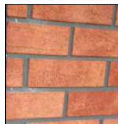
New Soltherm External Wall Insulation (Deco W-Brick ID) with brick cut render infills
