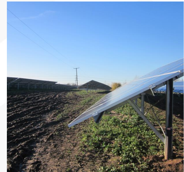
Figure 2.13: Example of a Solar PV Farm – the Vale of Glamorgan currently has 78MW of ground mounted solar PV installed
